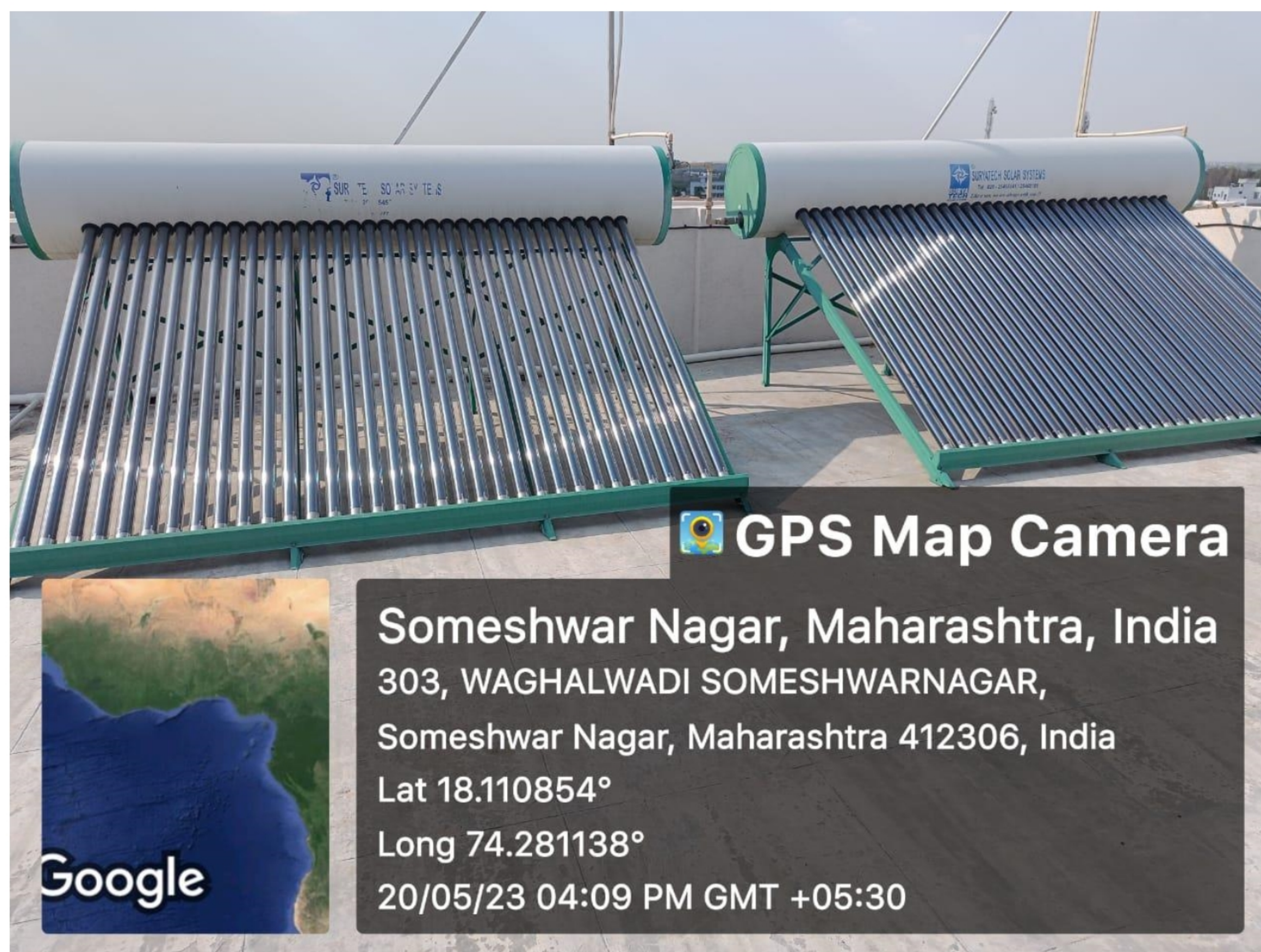
Solar Panel over Girl's Hostel
