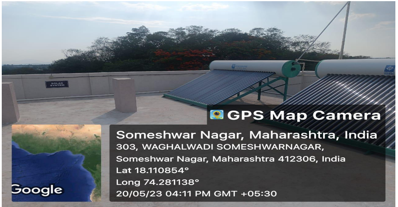
Solar Pannel For Hostel
