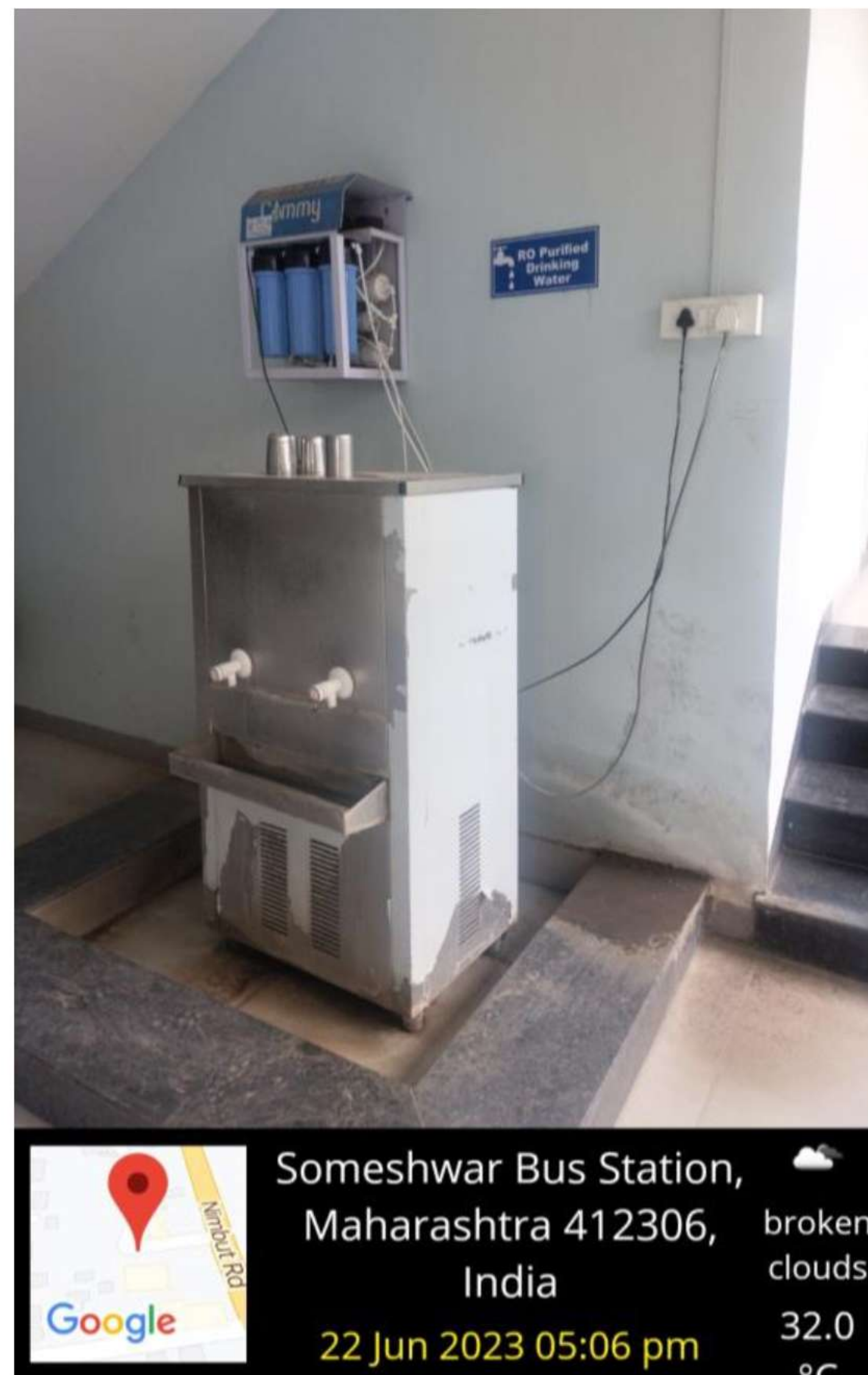
(R.O. water purifier in the college building)
