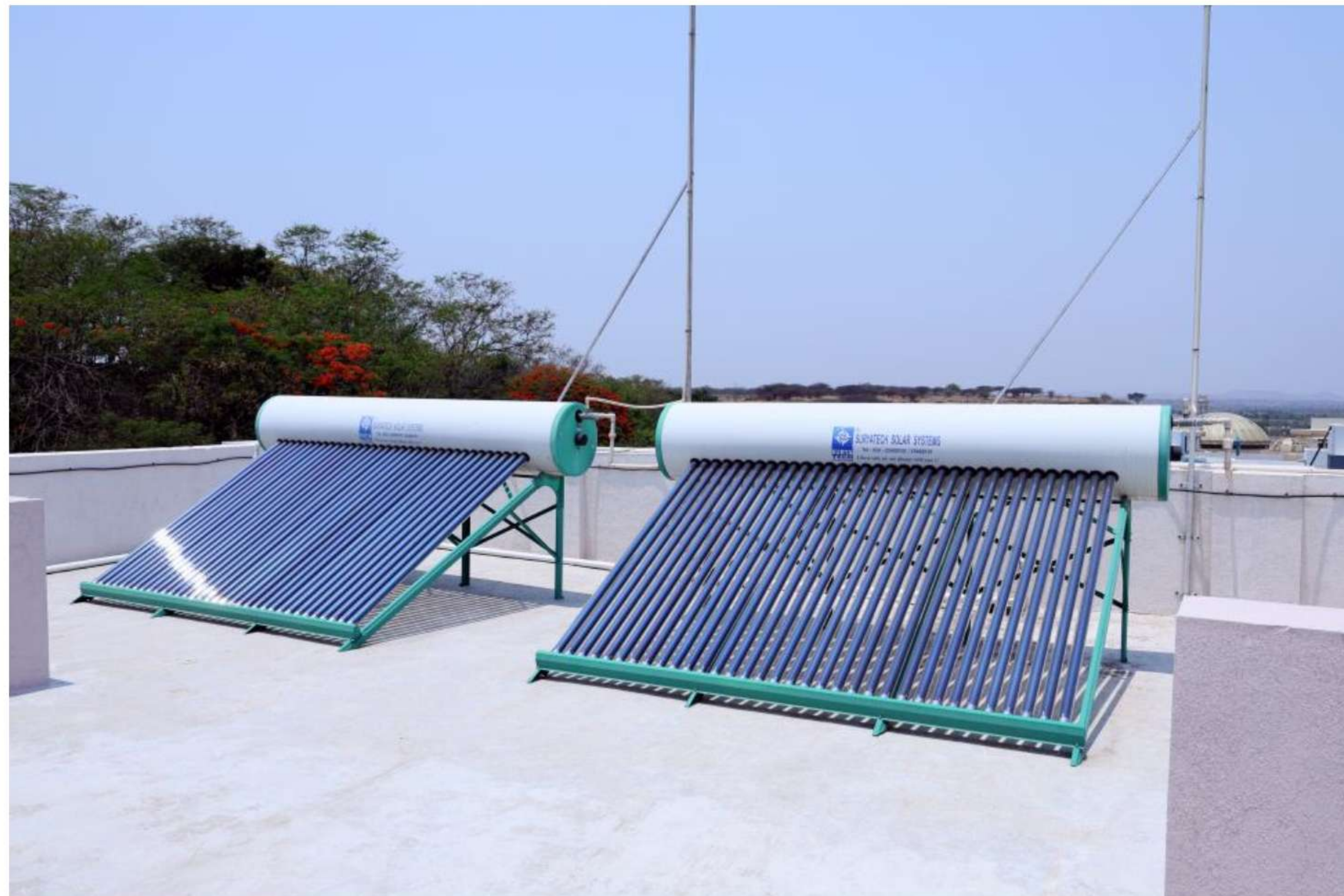
(4000 Liter/hour Solar roof top hot water system at girls hostel)
