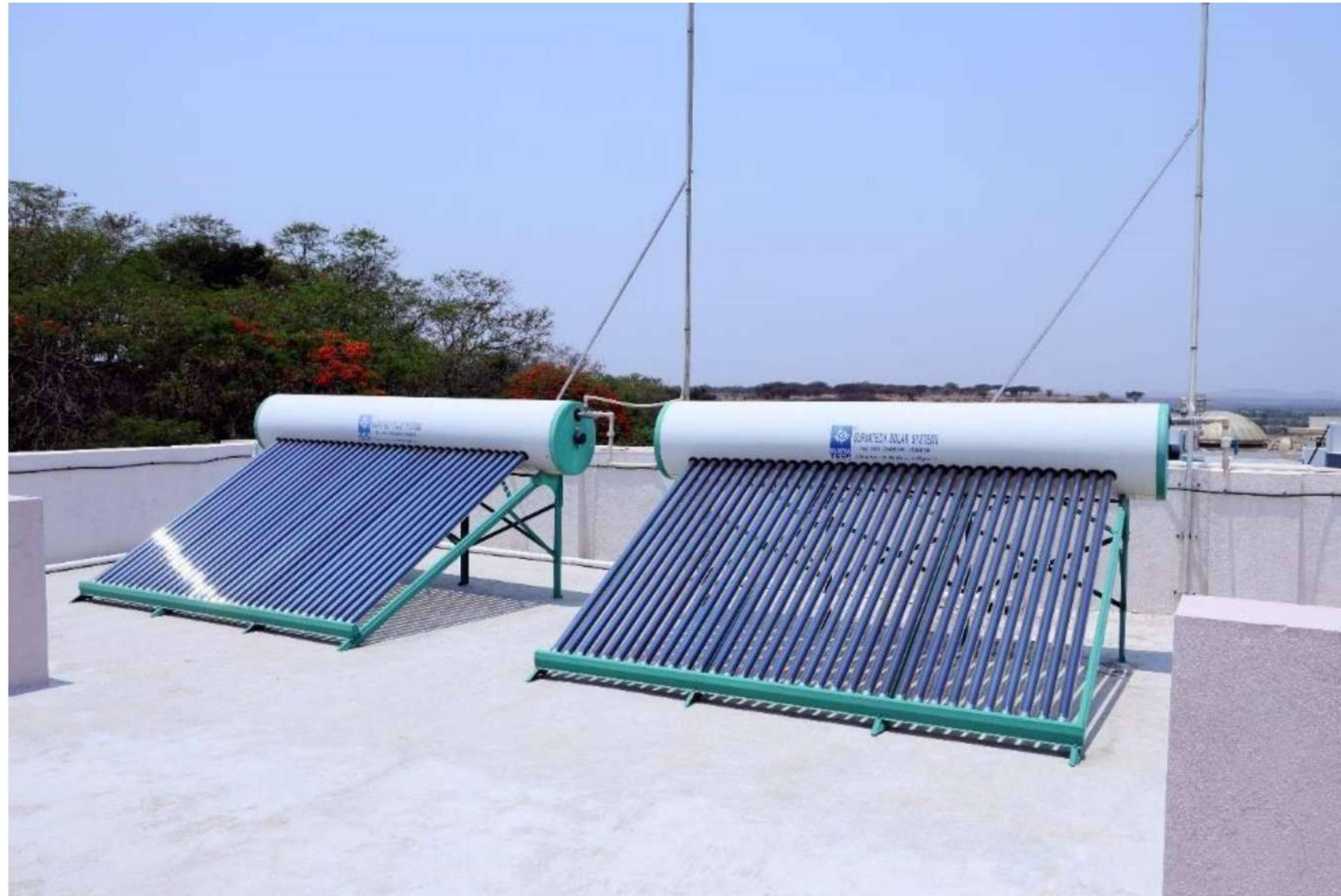
(Solar PV Hot Water Arrangement at Girls Hostel with Capacity: 4000 Liters per Hour)
