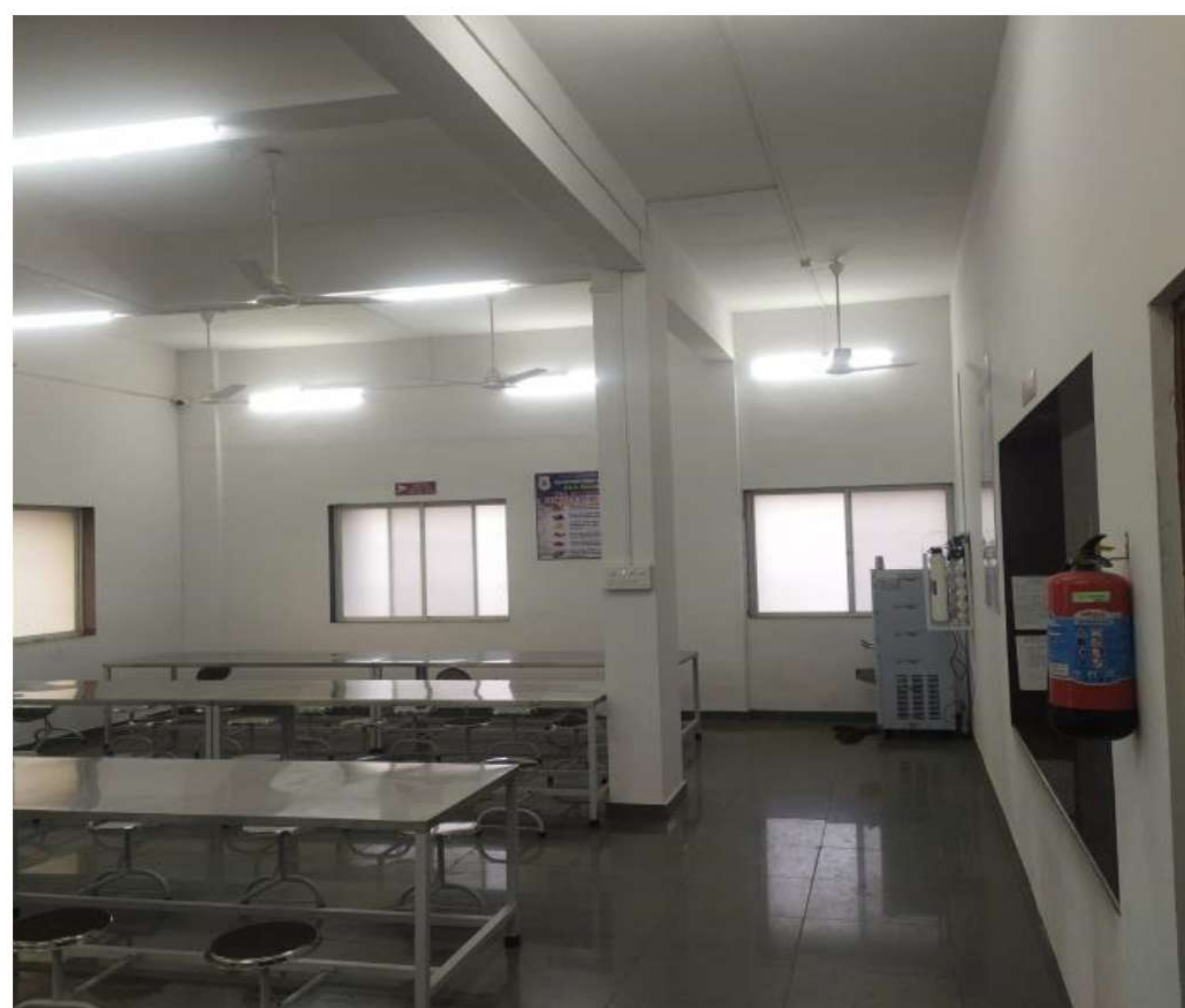
(BLDC fans and LED Tube Lights installed in the girls hostel )
