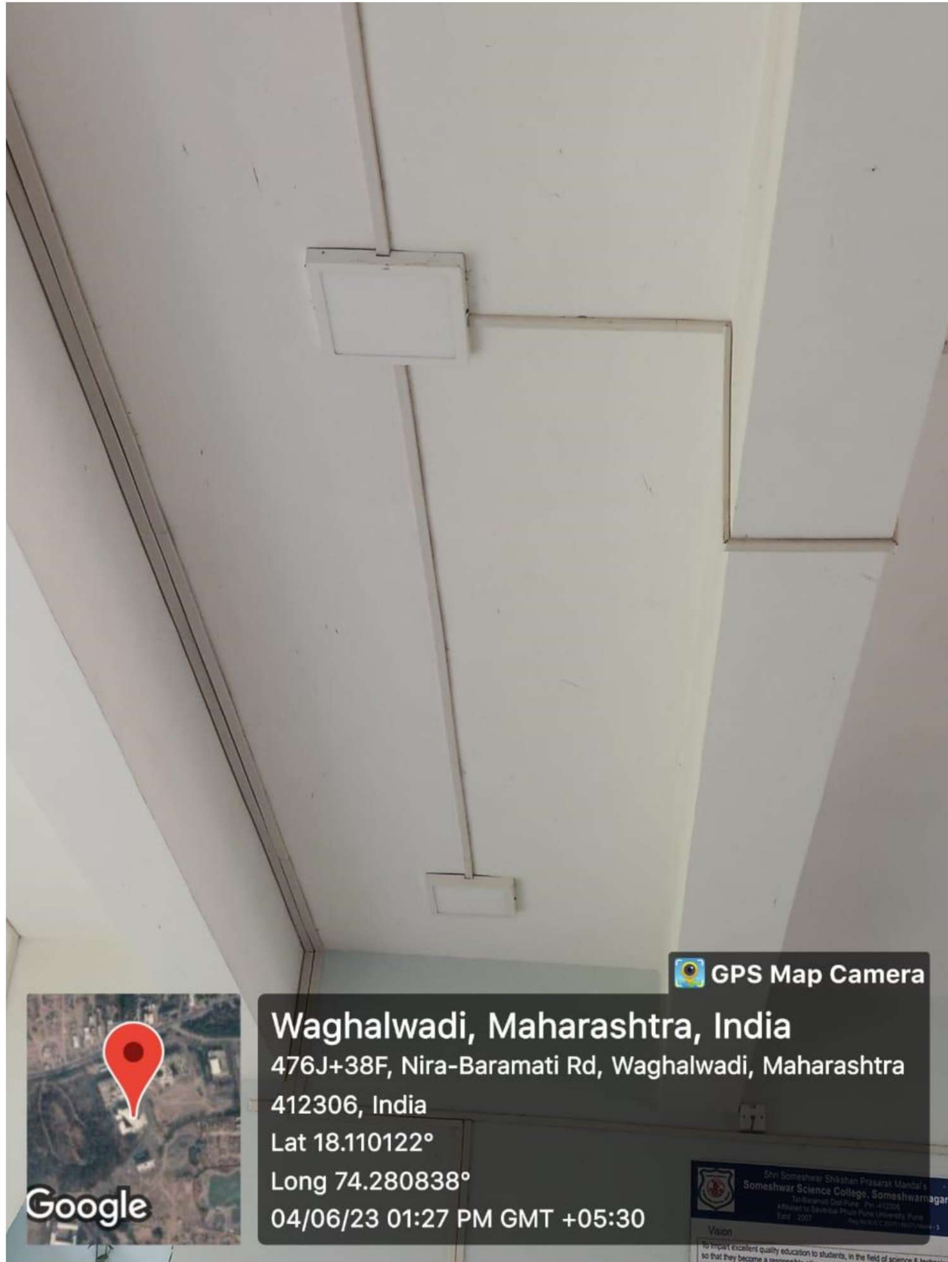
LED Lights (energy conservation) assembled in the open passage
