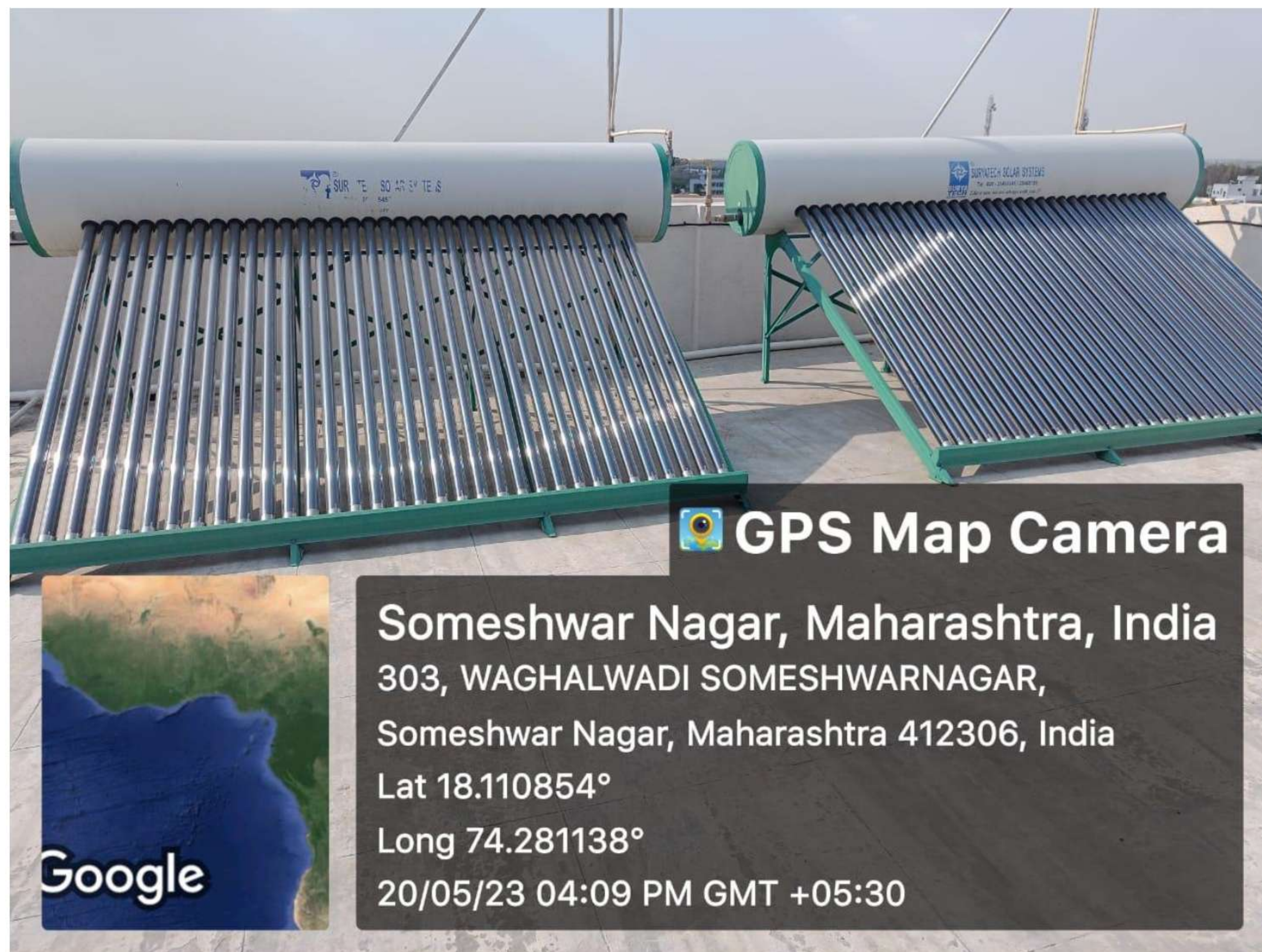
Solar Panels (alternate energy source) assembled over Girl's Hostel
